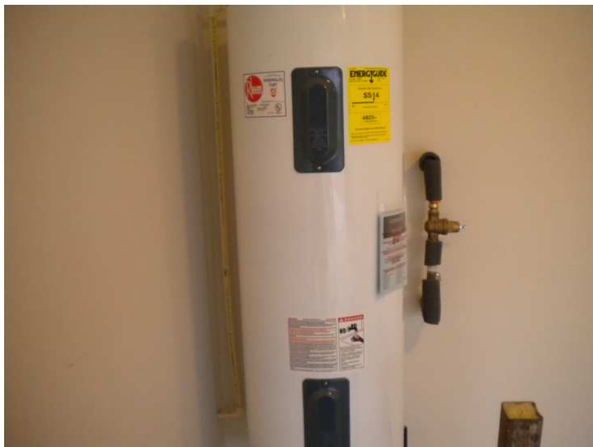
View of Water Heater
