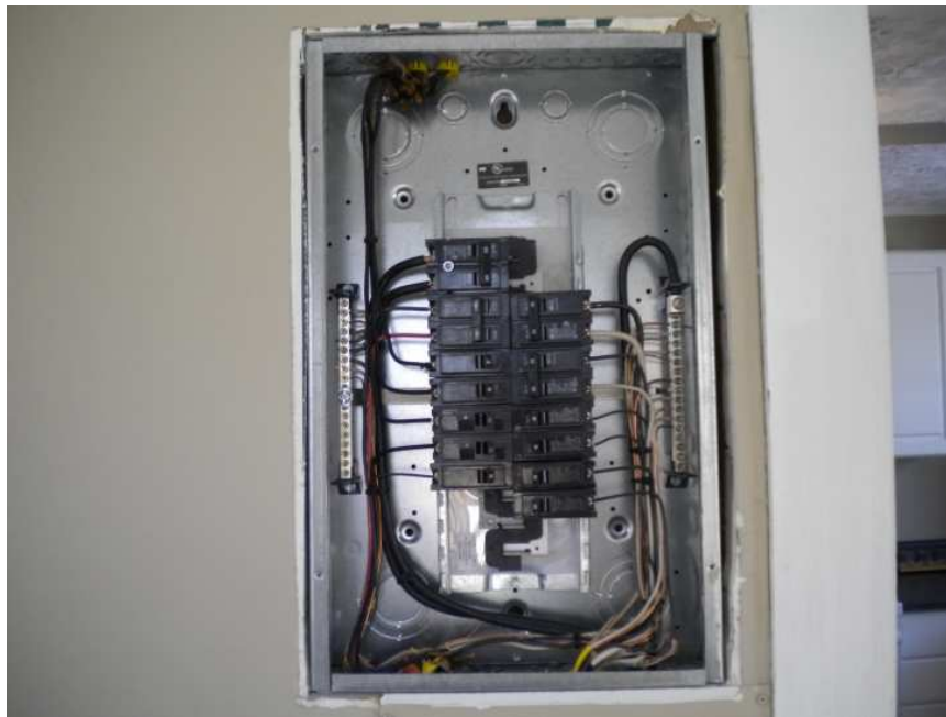
View of Main Electrical Panel
