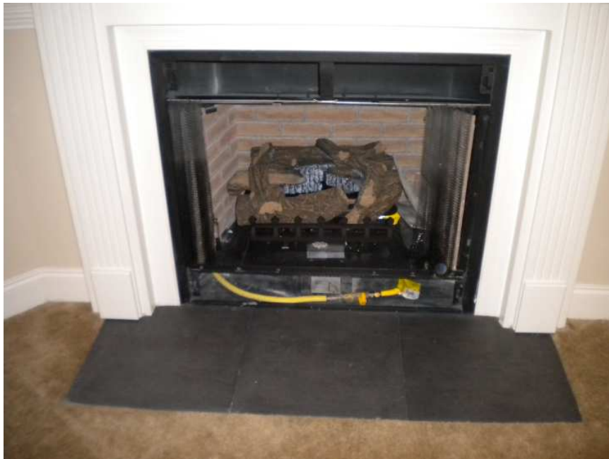
View of Fireplace@ Family Room
